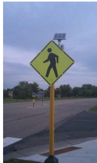
Figure 2 – Crosswalk Sign with Lights (after)
